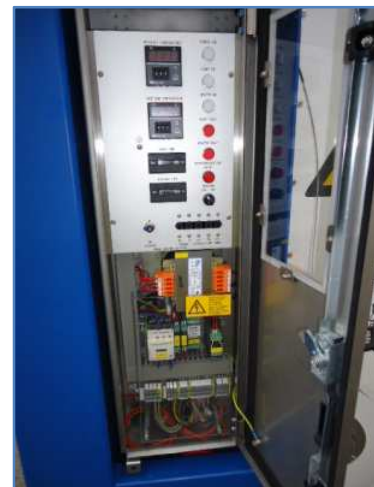
Hot water control panel
